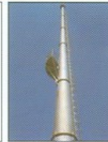
Self Supported Chimney
