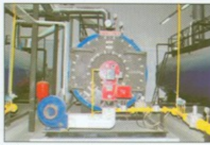
Hot Water Boiler
