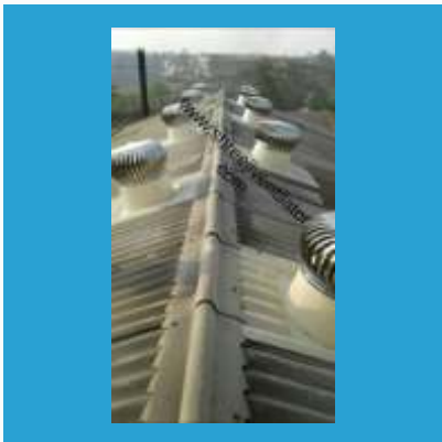
Roof Air Ventilator
