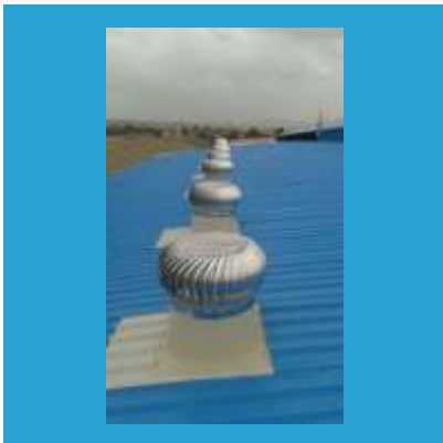
Roof Air Ventilator
