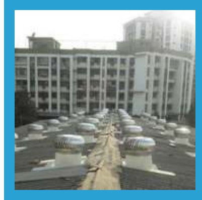
Roof Air Ventilator
