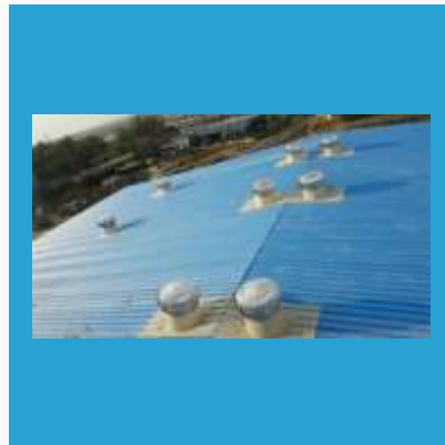
Roof Air Ventilator
