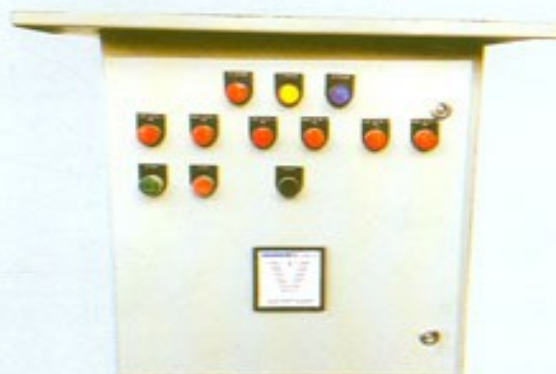
LEVEL SENSORS PANEL
