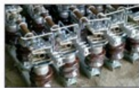
11 Kv Rotating Isolators
