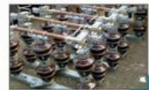
33 Kv 800 Amps Isolators
