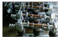
11 Kv 800 Amps Isolators
