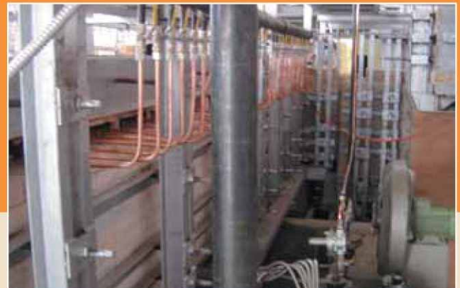
Glass melting furnaces
