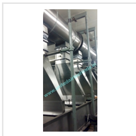
DRYING SYSTEM FOR CONVEYOR BELT
