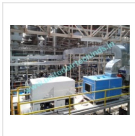
Industrial Fume Extraction System
