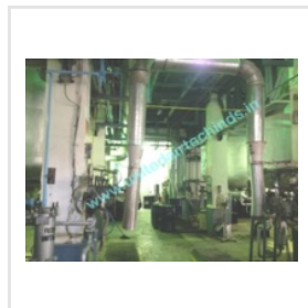
Industrial Air Ventilation System
