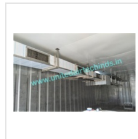
SS DUCTING WITH AIR VENTILATION GRILLS
