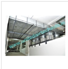
Paint Booth Exhaust System
