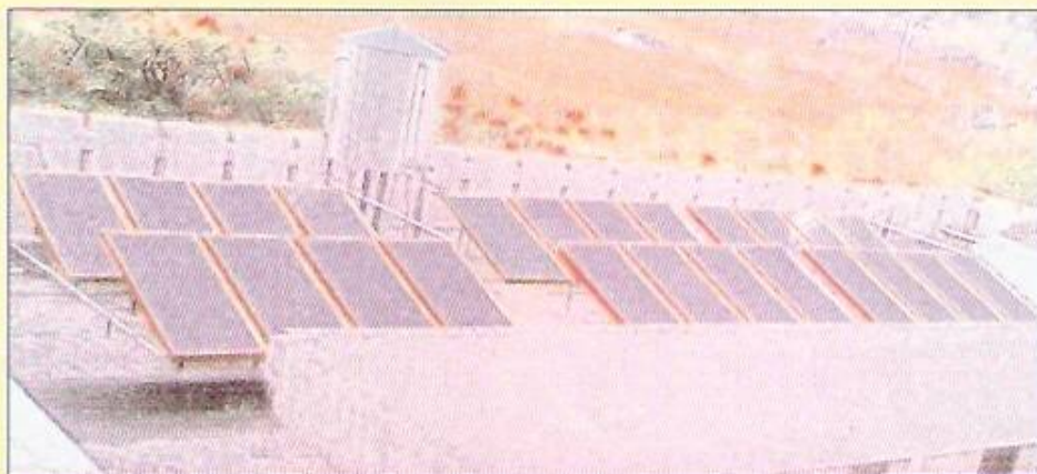
3000 LPD at Andhra Pradesh Police Academy
