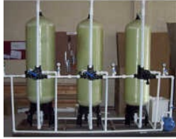
DM RO Water Plant Installation Service
